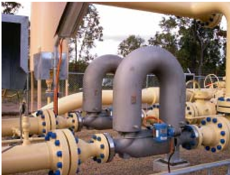
A 4" meter installed in 8" piping system
