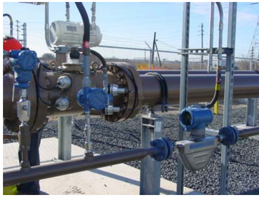
A ½” Coriolis and 12” ultrasonic in a fuel gas metering installation.
