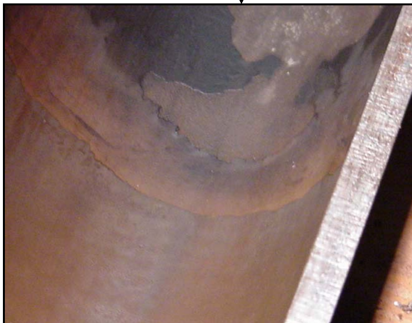
Figure 6 – Damage to internal plastic coating of joint C1 from exposure to high temperatures
