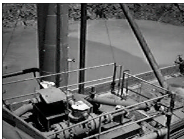
Figure 5 - Separator and manifold
