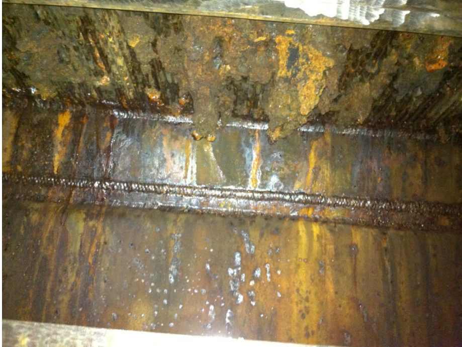
Figure 3. Gum formation plugging feed side channels. This is the area where the spray bars inject liquid into the channels
