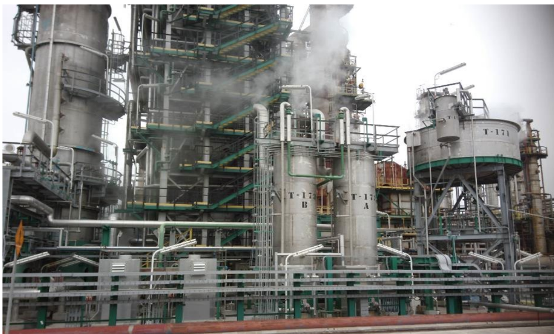
Figure 8 – BELCO® Purge Treatment Unit (PTU) at Bio Bio Refinery
