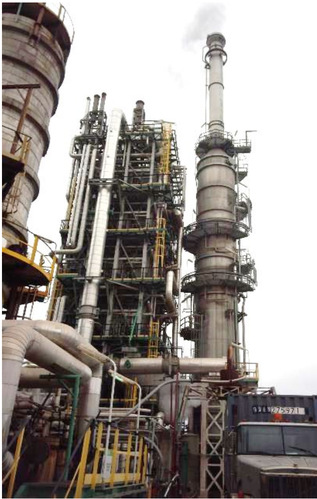
Figure 6 – BELCO® Scrubber Tower at Bio Bio Refinery
