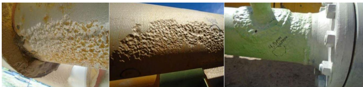
Figura 17: Zonas susceptibles a CUI I – Planta Solar
