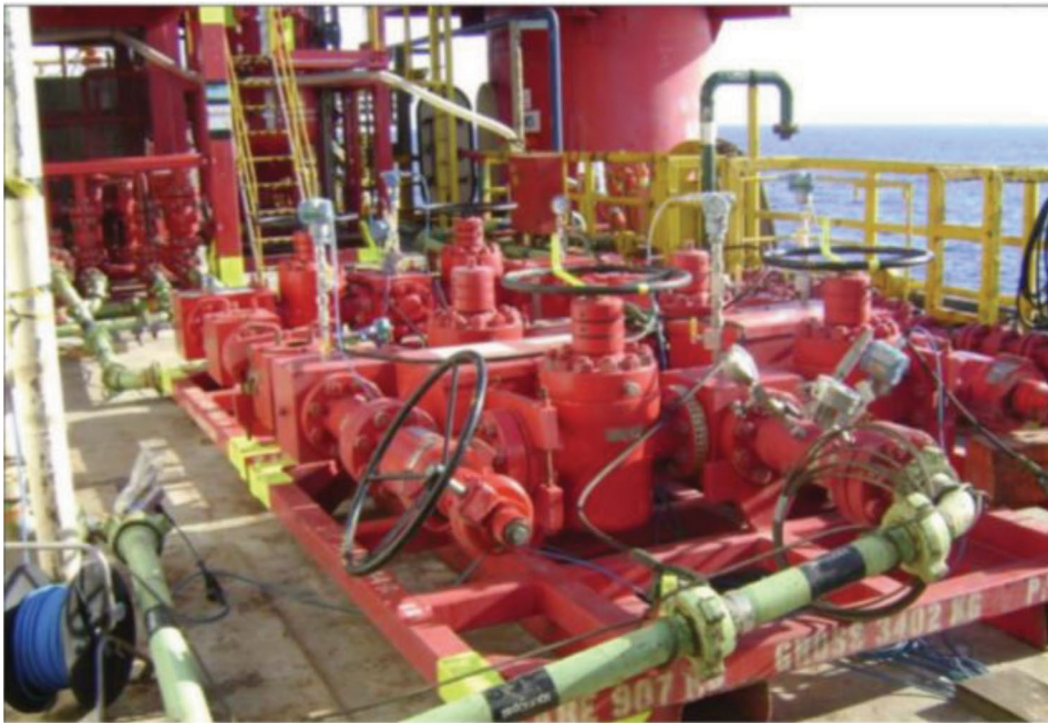
Figure 2. Frac Flow Back Choke Manifold
