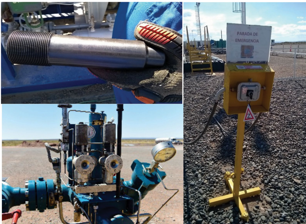
Figure 11. Restriction orifice (top left), SSV (bottom left) and ESD switch (right).
