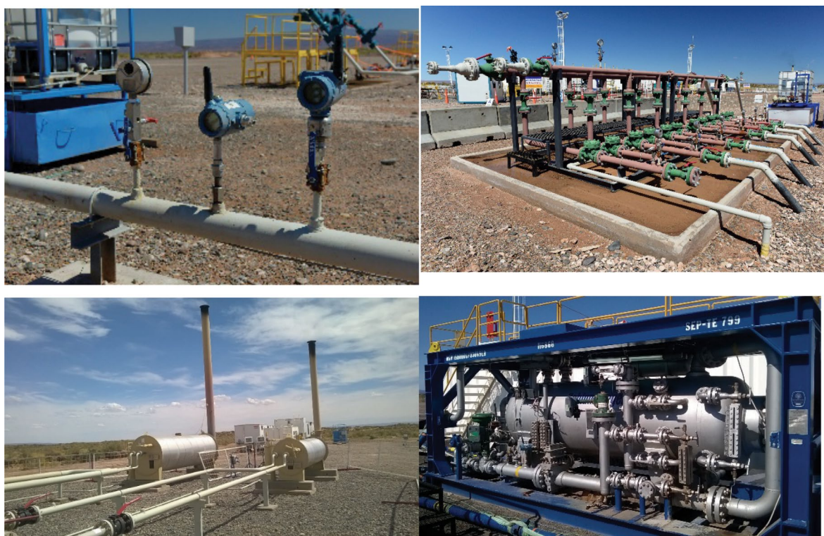
Figure 9. Data header (top left), field manifold (top right), heaters (bottom left) and separator (bottom right).
