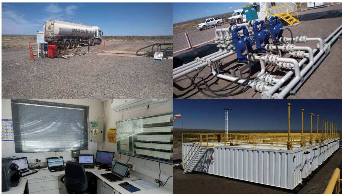
Figure 10. Loading station (top left), loading pumps (top right), data acquisition room (bottom left) and storage tanks (bottom right).
