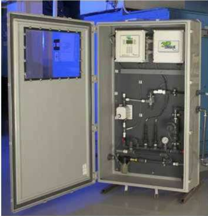
Figure 5 – Industrial 3D TRASAR Installation
