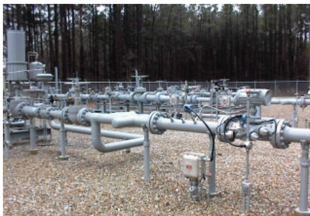
Three custody transfer meters from three suppliers plus three multi-regulator pressure reduction skids.....a lot of serious design considerations for one small site!
