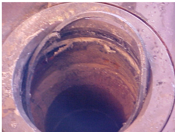
Figure 5. Damaged Choke Line Seals in Riser
